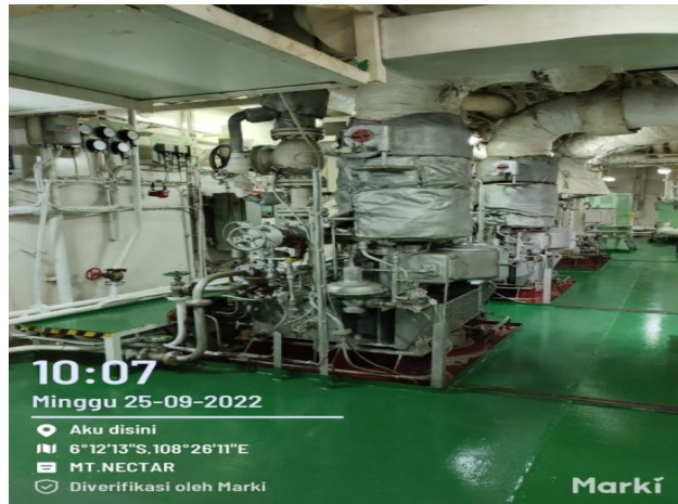
Gambar 1. Cargo Oil Pump Turbine
